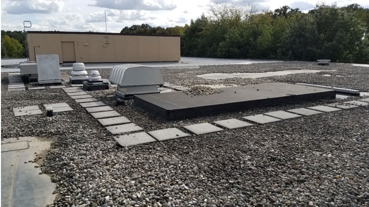
Von Ohlen Hall Roof - Facing Southwest from VON Roof (view of abandoned curbs to be removed):
